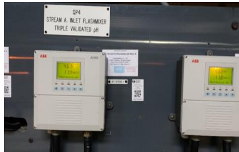
Figure 2: Analysers for pH triple validation at the inlet works
